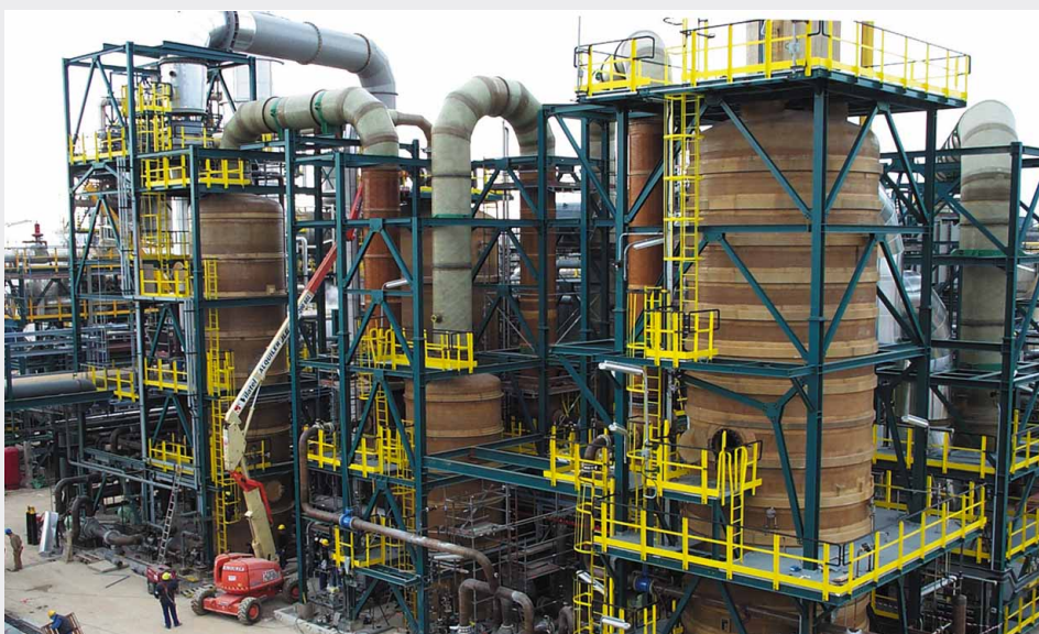
Overview of the Dynawave plant in Tarragona - Spain.
