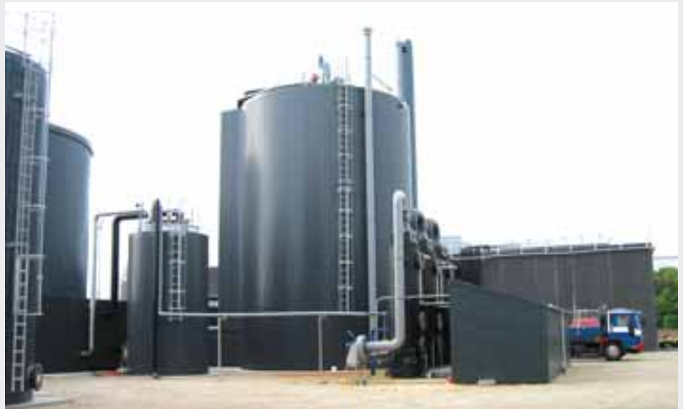
Biological waste storage according to the new Tunetanken concept
