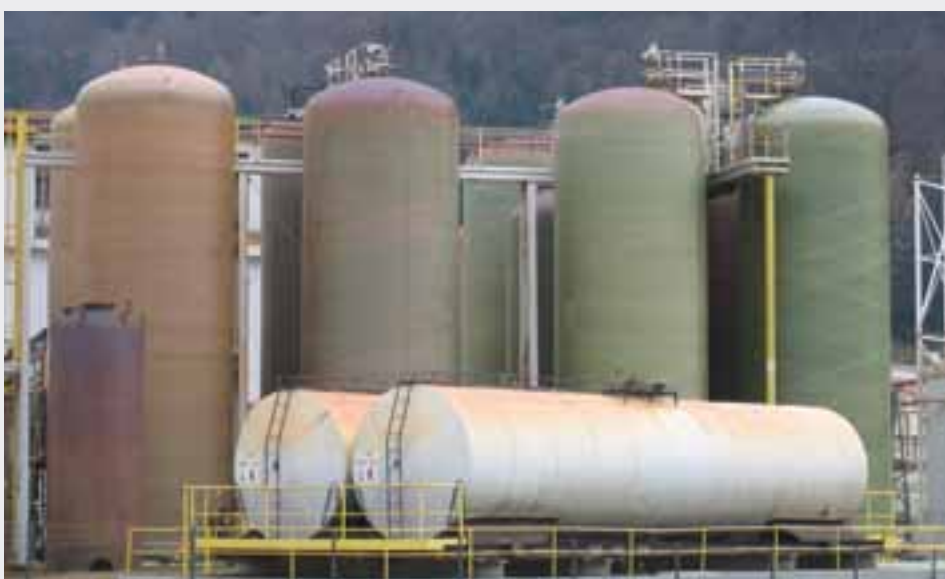
Strong acid storage tanks.
