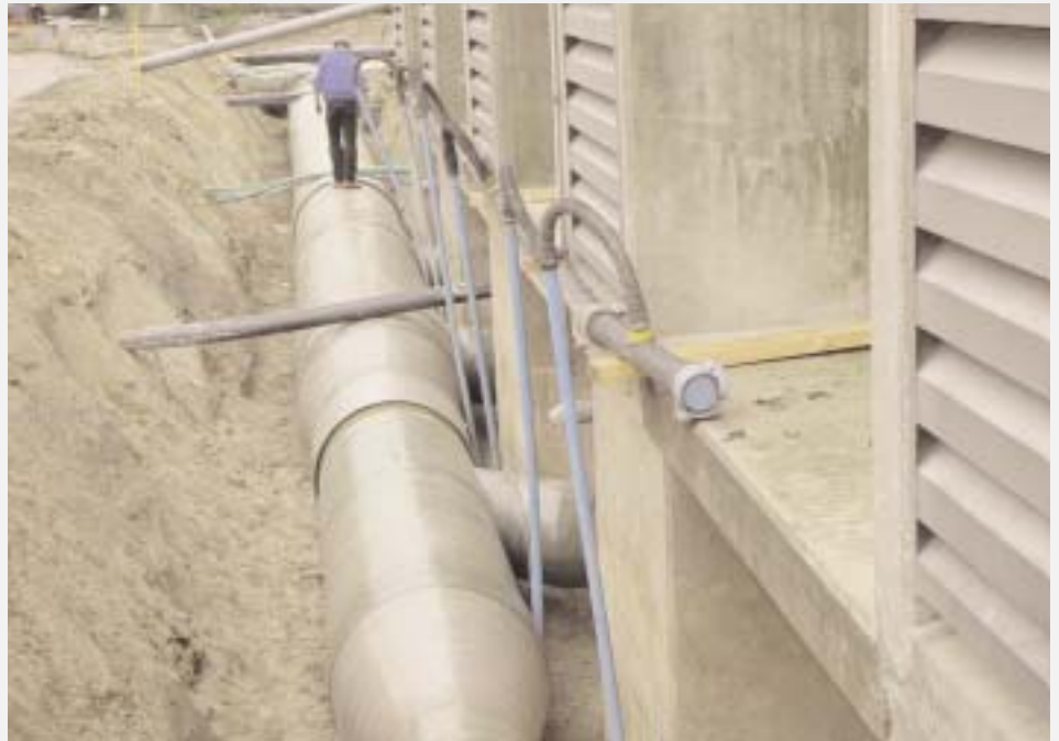
Newly installed hot air pipeline
