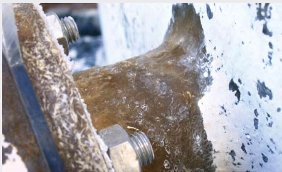
Alkaline corrosion problem at flange due to caustic soda attack
