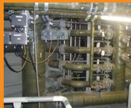
FRP pipe lines
