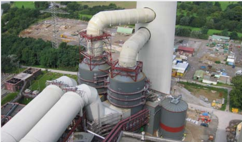
Atlac FRP piping at powerplant
